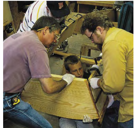
From left to right, Hott, Merlin, Lars and Eisenlord wrestle the assembly of the sides, stem and transom into shape with a temporary spreader to hold the shape of the hull. As you can see, it takes all hands on deck to pull these parts together.
